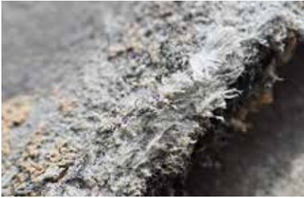
Pictured: Close-up of asbestos in building material. Source: Supplied.
